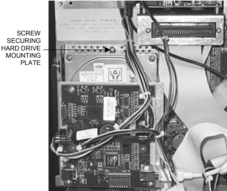
FIGURE 10 - TOP VIEW OF I/O BOARD AND HARD DRIVE
